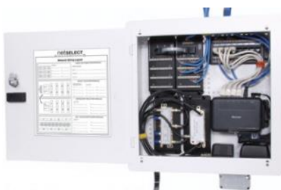
Figure 25 Residential Wiring Cabinet
