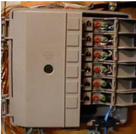
Figure 26 Typical Telco Demarc
